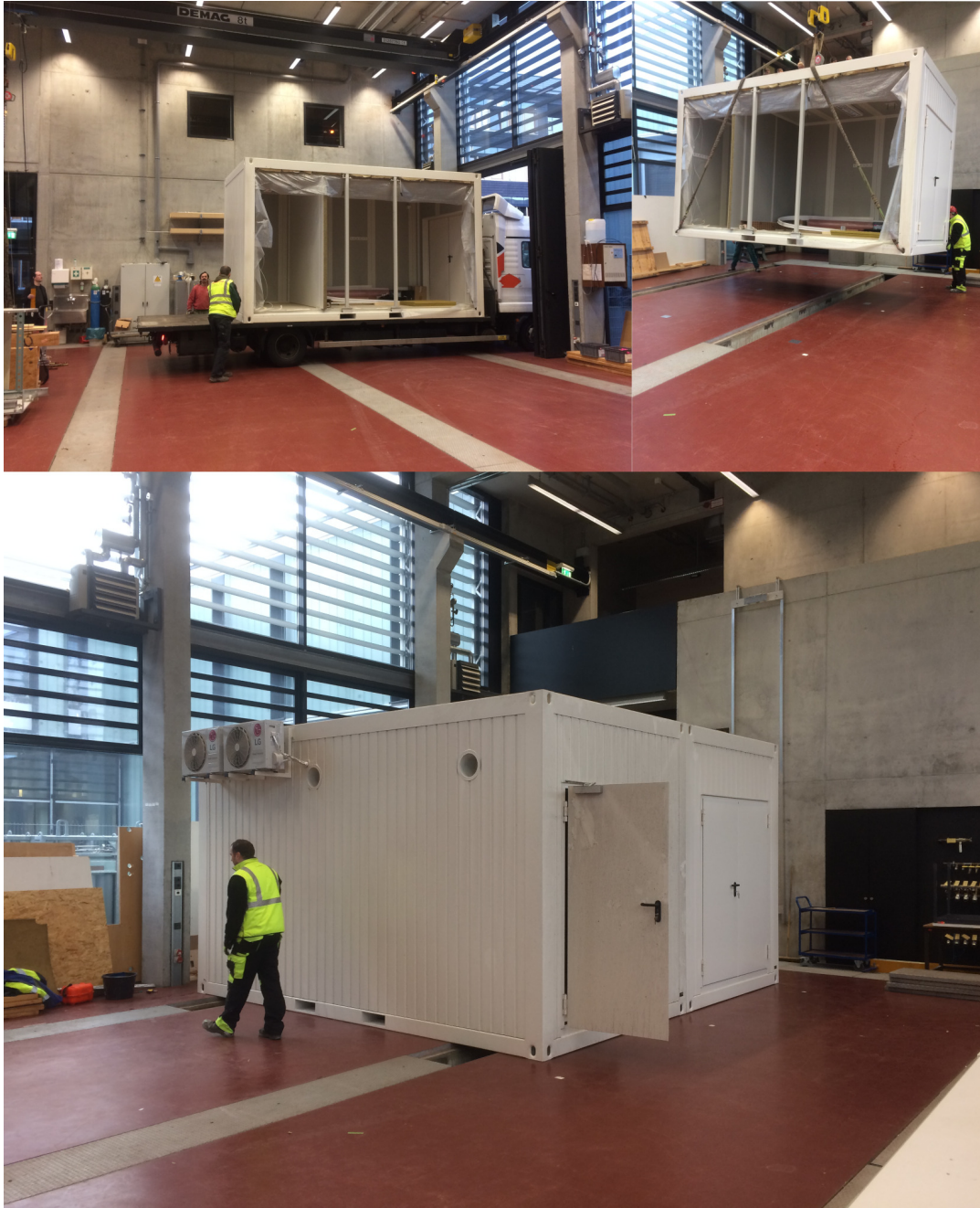
FIGURE 4.3: Photos of the delivery and setup of the laboratory container. The manufacturer Algeco delivered the two parts of the container on trucks. The crane inside the experimental hall, operated by our mechanical workshop, moved the pieces to the designated location. A construction team from the company assembled both parts mechanically, connected the electrical wires and laid the floor with the cut-outs over the cable ducts. After two days, the container was ready for a final product inspection and approval.
